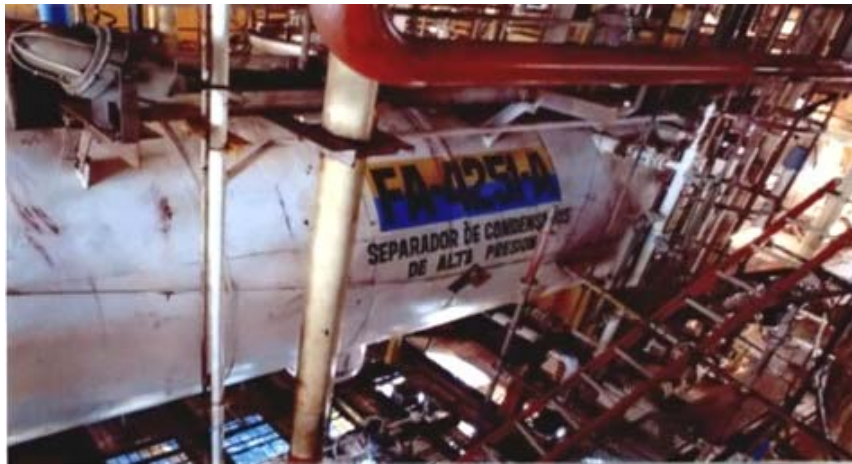
Figure 2: Photograph of the assessed pressure vessel installed and operated in an oil production offshore facility.
